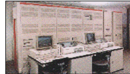
Central Office Switch
